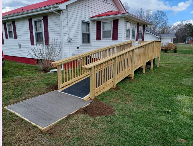
An example of the wheelchair ramps FTAAAD is constructing with funding through the Options 2.0 program
